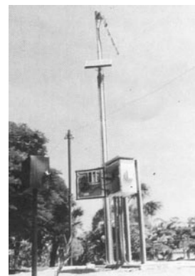
Figure 9. Field measurement site of the telemetry system
